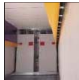
4 High-volume air flows into side plenums, which — when the trailer is loaded — creates a high-pressure zone, resulting in uniform air flow and temperature throughout the cargo.
